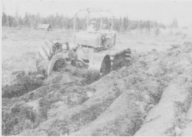
Fig. 6. Land clearing in a bog with a thick layer of peat. Allis-Chalmers HD 5 track-type tractor equipped with wooden shoes bolted on tracks. A large Fiskars-model land clearing plow used for ploughing.
