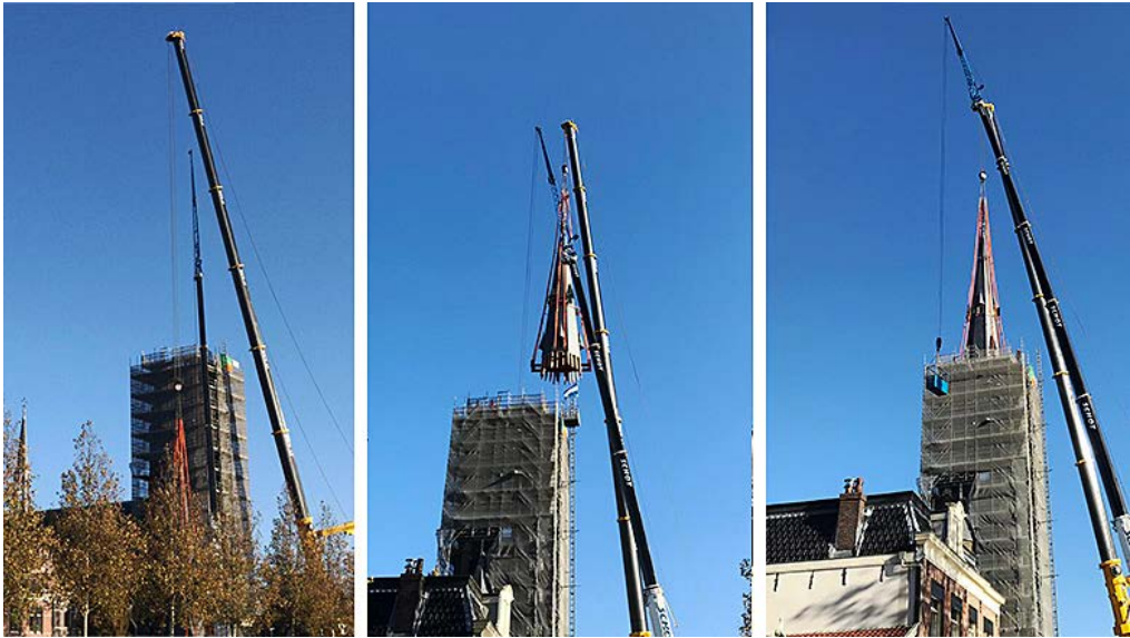
The new spire being placed on the Saint Laurentius Church, 8 November 2016. Photos by NH.
