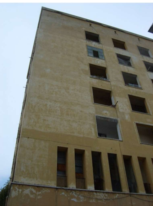
Figure 18. Former Casa del Fascio and police station, Quarticciolo. The upper floors have been converted into apartments. Photo: author (2018).
