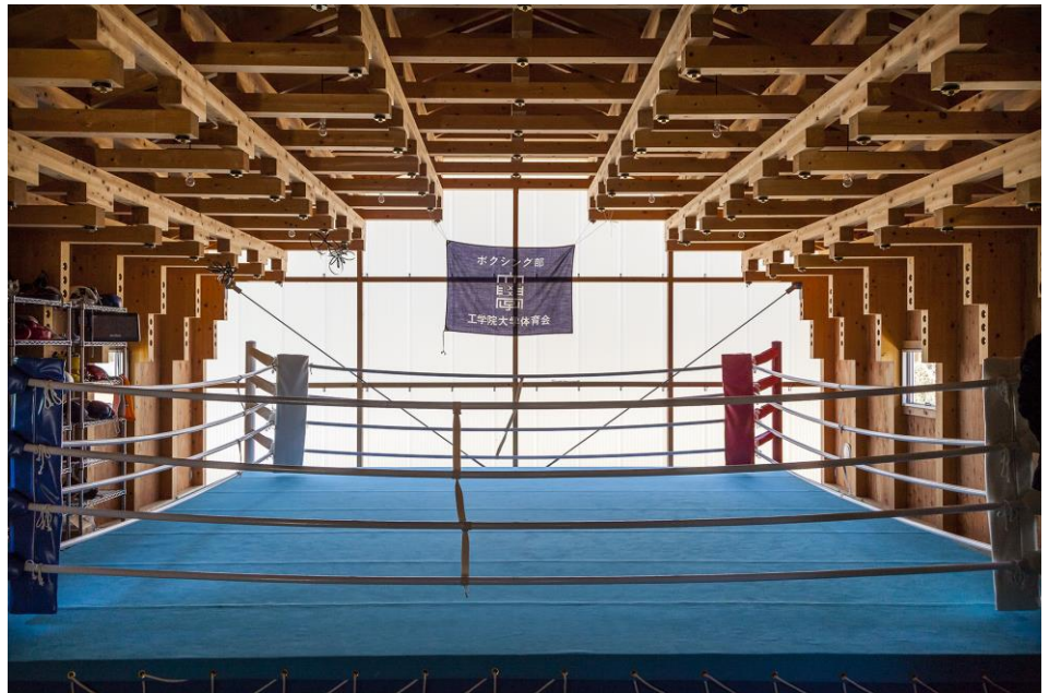
Figure 20. Use efficient forms for long spans from short pieces. Although not made of reclaimed timber, this figure illustrates the 5th principle with the corbelled roof structure of Kogakuin University Boxing Club in Tokyo, designed to be built from short low-quality wood (designed by FT Architects, photo in the courtesy of Jonas Aarre Sommarset).
