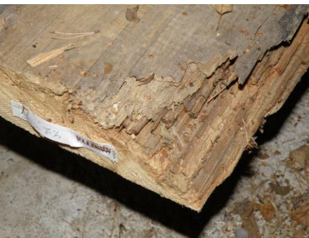
Figure 8. Rot at the end of a salvaged floorboard. Damage in wood is easy to recognize visually.
