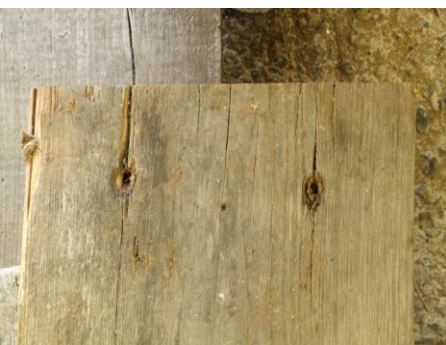
Figure 15. Cracking and nail holes at the end of a floorboard.
