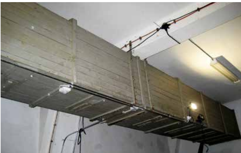
Photo 45. The ventilation shaft where the German documents were found. Photo Jan Fast.
