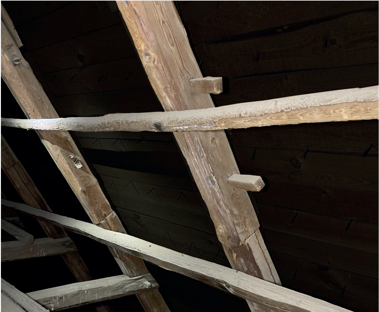
Figure 4. The rafter extension in the nave roof structures of Ulvila church. Photo: Laura Laine, edited by Franziska Dalheimer.
