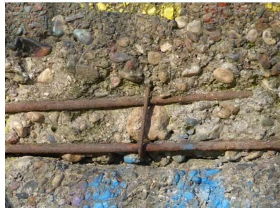
Figure 2: Schoolyard, detail: old concrete with steel bars exposed.
