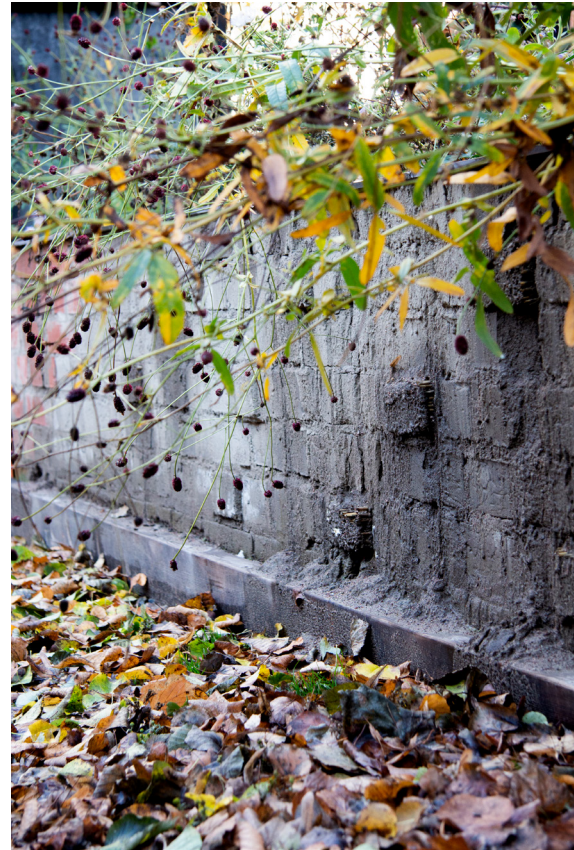
Figure 12: Raw clay bricks erode as rainwater washes over them. Great Burnet ( Sanguisorba officinalis ). Alusta Pavilion. October 2022. Photo: Elina Koivisto.
