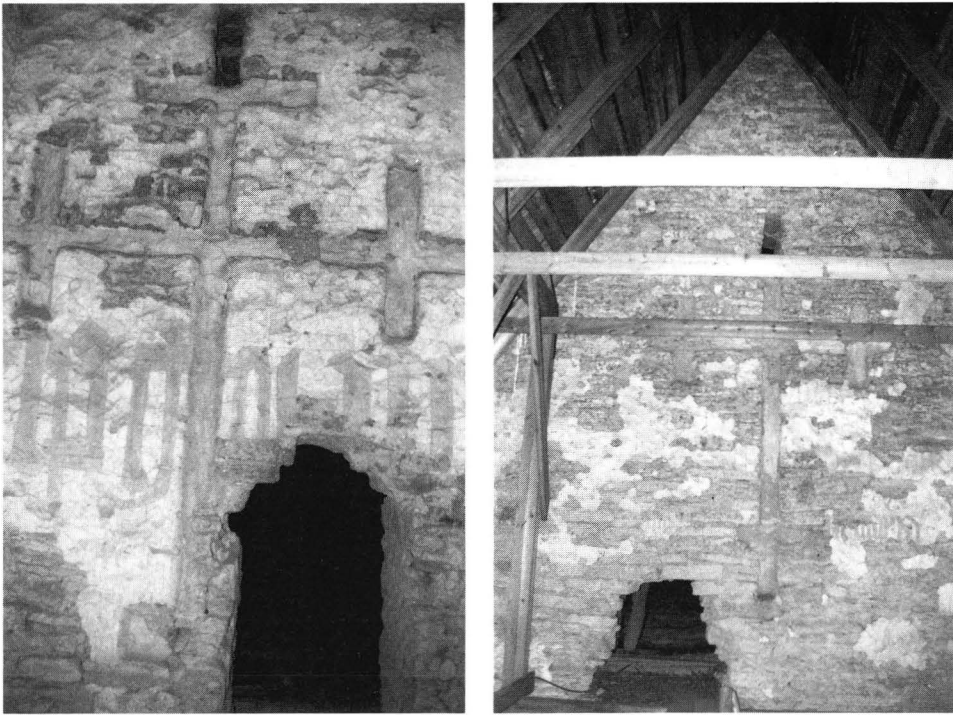
Fig. 7. The Church of Lügänuuse, nave. Crosses of the west (a) and east (b) gable ends and text fragments on plaster and whitewash. — Photos MH 31.3.1990.
