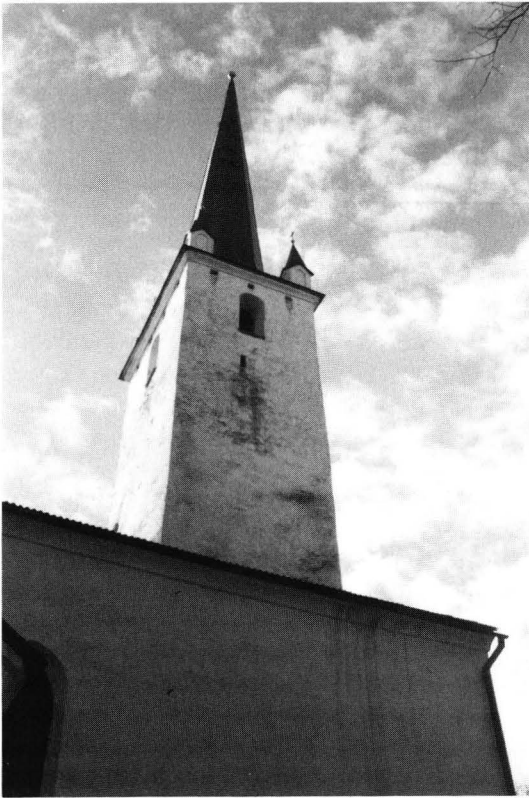
Fig. 20. The tower of the Church of Ambla, NNE view. The tower rises from the westernmost vaulted part of the nave. The bell-storey was built after the Middle Ages. — Photo MH 1. 4. 1990.
