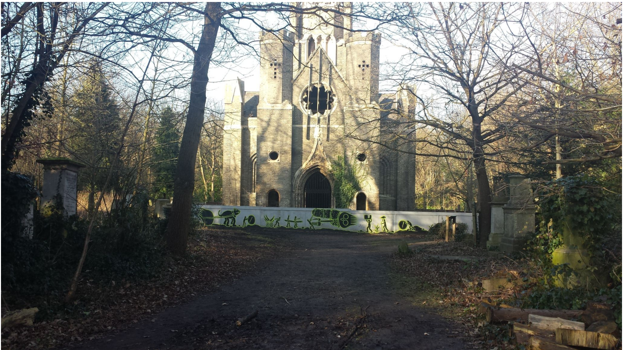
Photo 4. Abney centre chapel in partially ruinous state at the beginning of renovation. Photo: Romany Reagan, 2015.
